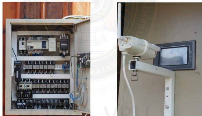
a) control box
